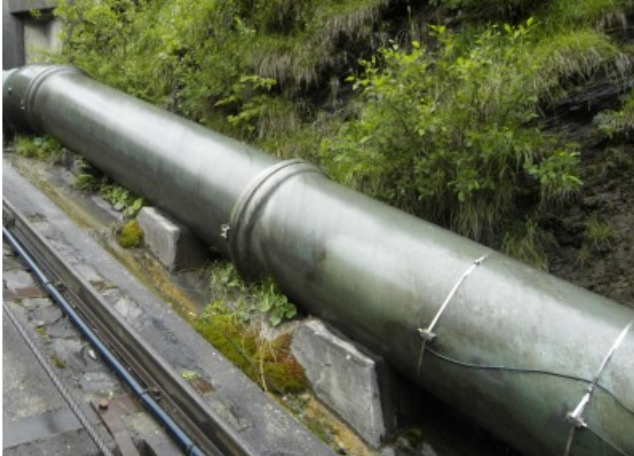
Turbine intake flow measurement using clamp-on sensors
